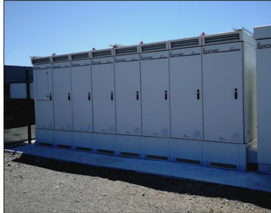
Typical centralised inverter
