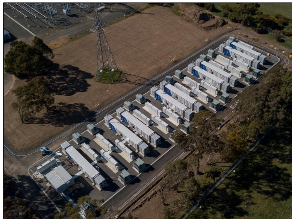
Typical battery storage compound configuration
