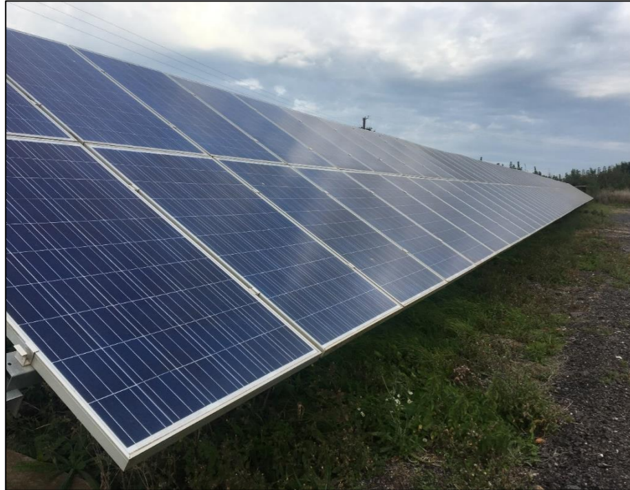
Typical solar panels
